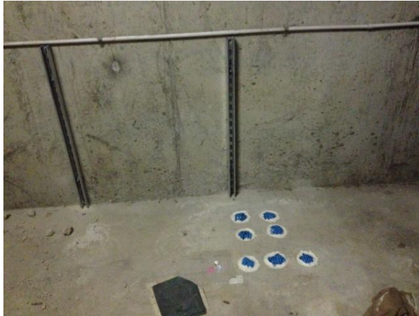
Plantroom showing cored holes with temporary firestopping and vertical Flexistrut rack to which your pipework will be clamped.
