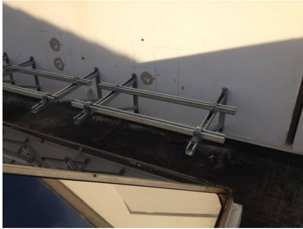
Condenser bracket. The bars can be adjusted to suit the “feet” of your condenser. Cored holes for pipework that have been temporarily firestopped are also shown.
