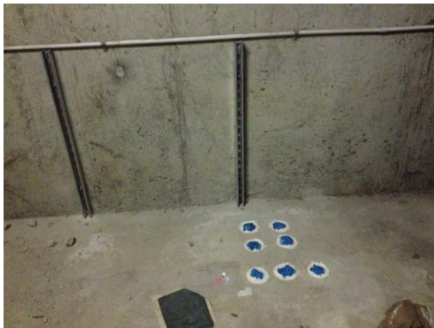
Plantroom showing cored holes with temporary firestopping and vertical Flexistrut rack to which your pipework will be clamped.
