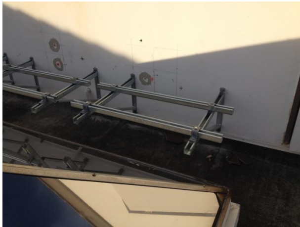
Condenser bracket. The bars can be adjusted to suit the “feet” of your condenser. Cored holes for pipework that have been temporarily firestopped are also shown.
